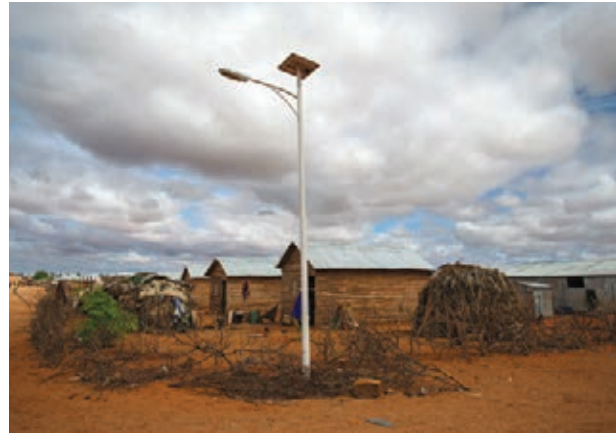
Image 43: A solar-powered streetlight provided by IKEA Foundation stands in a refugee community in Kobe camp. © IKEA Foundation/Åsa Sjöström, 2013
