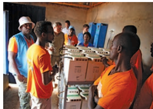
Image 21: Energy cooperative members in Buramino show visitors the equipment used to store energy generated by the solar panels. © UNHCR, 2019
