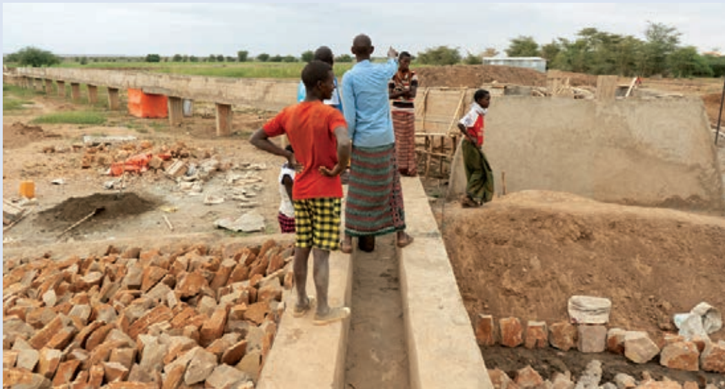
Image 60: A team of builders finalise the concrete irrigation canal in Hilaweyn II. © RSC/Raphael Bradenbrink, 2018
