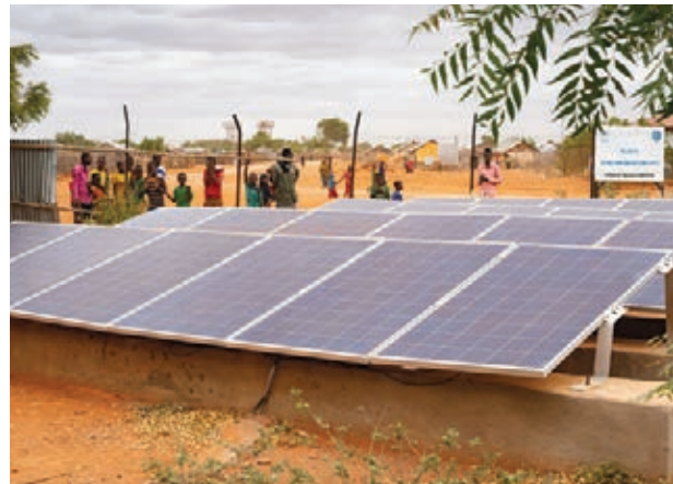
Image 42: Solar panels maintained by the energy cooperative power the ARRA-run health centre in Hilaweyn camp. © RSC/Raphael Bradenbrink, 2019
