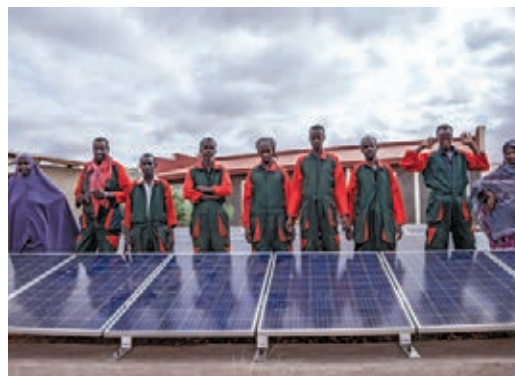
Image 4: Refugee and host community technicians in the energy cooperative stand with a recently installed solar mini-grid. © UNHCR/Diana Diaz, 2018
