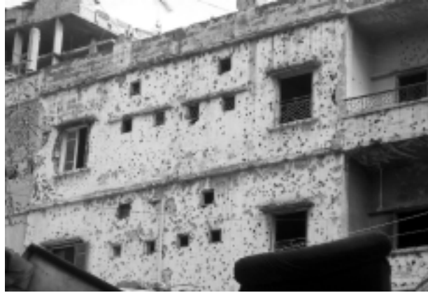
War-damaged building at refugee camp Bourj el-Bourajneh, Beirut. (E. Vasta/S. Castles)
